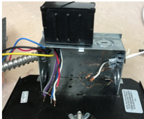
Figure G: Load cable and controller within junction box.
